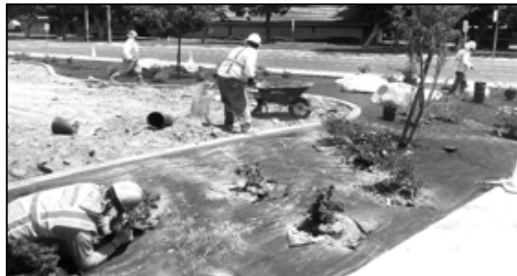
MAHAM MEMON/The Shamrock Construction workers working at the front of campus during the final phase.
